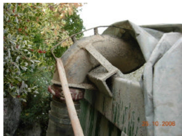
Figure 12: drain off the cuttings into a hutch using a safe transportation hose
