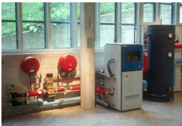
Figure 17: GSHP in the museum of natural history in St. Gallen, Switzerland (photo from 1993)
