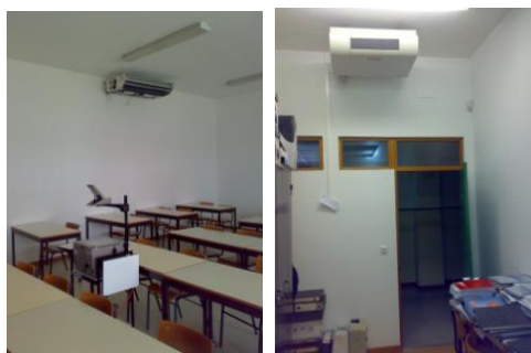
Figure 7: Terminal units, fan-coils, in one classroom and in one office
